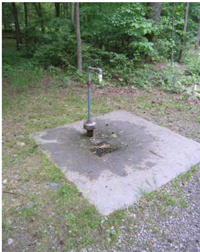
Figure 9.6. This spigot is not a frost-free design, but the facility has a good drainage system and hardened surface around the concrete slab that prevents formation of a mudhole. (See frost free design in Figure 9.9.) (Photo by G. W. Wood.)
