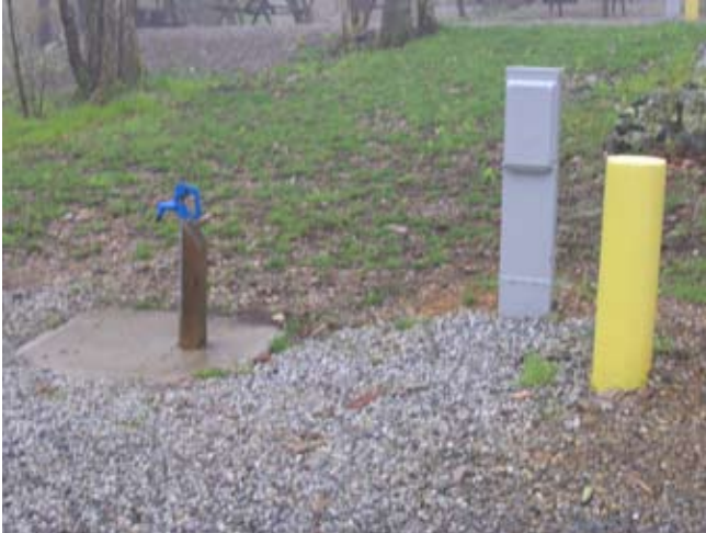
Figure 9.9. An electrical hookup with an adjacent concrete post to prevent damage by moving vehicles. The frost-free water spigot is located about 5 ft. downslope of the hookup device. This proximity of the water facility to the electrical facility is apparently acceptable to design standards in Virginia. This would not be a suitable place to shower a horse. (Photo by G. W. Wood.)
