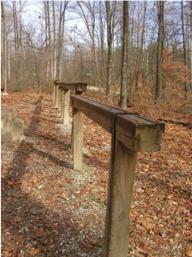
Figure 9.24. A hitching rail with edges covered by angle iron for protection from chewing. If a horse should get up on this rail, a disaster is eminent. (Photo by G. W. Wood.)
