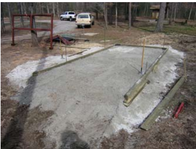
Figure D.18. Pressure-treated 4x6 timbers in the floor framing on three sides with one end left open to allow equipment to set the central divider in place. (Photo by G. W. Wood.)
