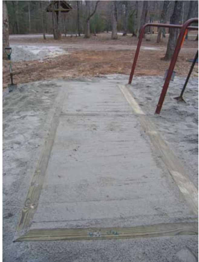
Figure D.14. Floaters (2x6 pressure-treated timbers) placed on 48-in. centers and even with surface of floor fill material, floor framing, and center support beam. (Photo by G. W. Wood.)
