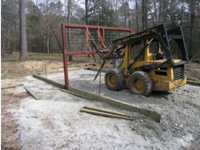
Figure D.19. Use of a skid steer to set the central divider into place. (Note that the divider is secured to the skid steer forks with a rope for personnel safety reasons.) (Photo by G. W. Wood.)
