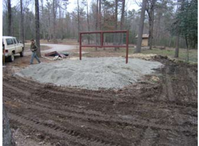
Figure D.20. Quarry screenings fill the stall floor area and embank its perimeter to eliminate sharp drop-offs. (Photo by G. W. Wood.)
