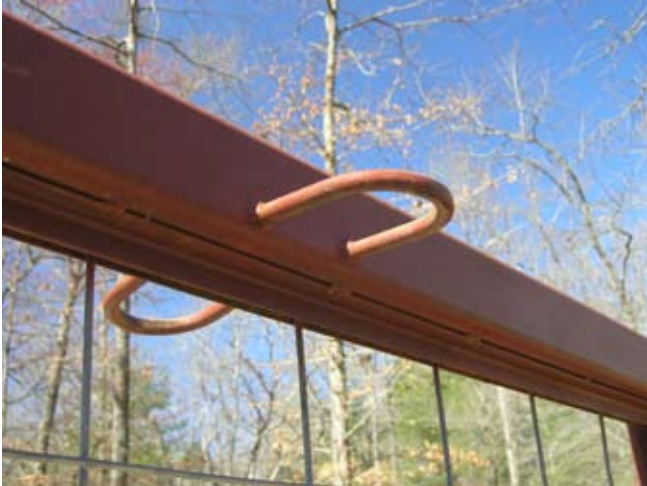
Figure D.6. The \frac{3}{8} -in steel rod tie-bolt welded on the top horizontal member of the central divider. (Photo by G. W. Wood.)
