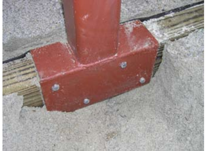
Figure D.4. The 3\frac{1}{2} - x 12-in., three-sided sleeve at the bottom of the central divider upright attaching the central divider to the framing timbers. Fasteners are \frac{3}{8} - x 2 \frac{1}{2} -in., galvanized lag bolts (GHD if available) located both inside and outside of the framing timbers. (Photo by G. W. Wood.)
