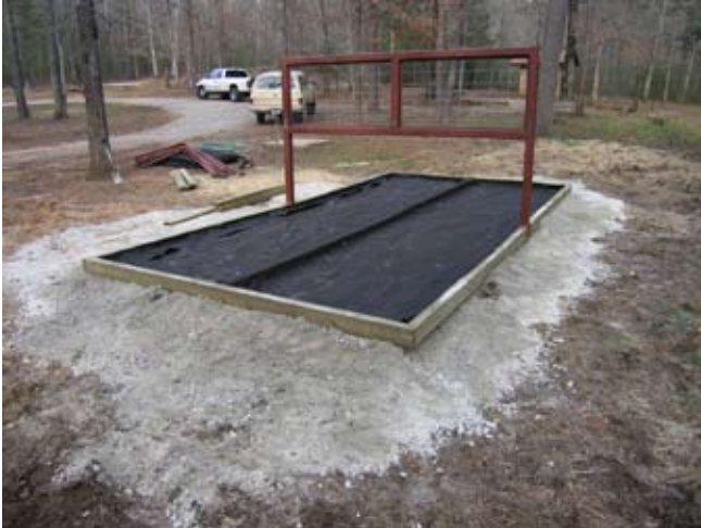
Figure D.13. A 5-oz. geotextile liner separating the floor fill material from the crush-and-run gravel foundation. (Photo by G. W. Wood.)
