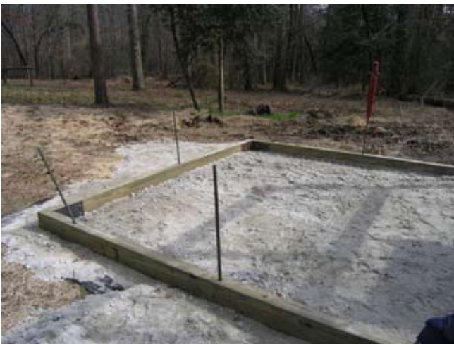
Figure D.11. Anchoring rods ( \frac{3}{8} -in. rebar, 5 ft. long) ready for driving in framing timbers. The two slanted anchoring rods for the end timber are not shown here. (Photo by G. W. Wood.)
