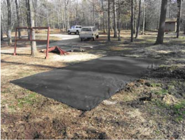
Figure D.16. The 5-oz., non-woven geotextile ground liner fastened around the perimeter with 6-in. wire staples. (Photo by G. W. Wood.)
