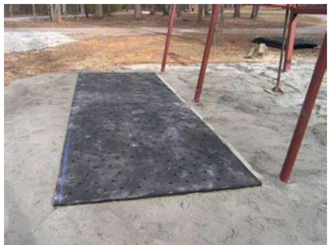
Figure D.15. Placement of perforated stall mats fastened to floor framing and center support beam timbers with 1½-in. deck screws. (Photo by G. W. Wood.)
