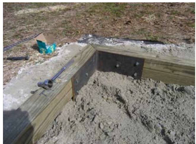
Figure D.12. Joining the floor framing corners with steel strap ( \frac{1}{4} x6x24 in.) bent to 90° and fastened with \frac{3}{8} - x 2½-in., galvanized lag bolts (GHD if available). (Photo by G. W. Wood.)
