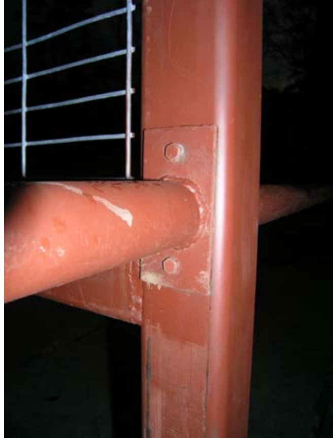
Figure D.7. Attachment of the stall rail to the central divider with \frac{3}{8} - x 1-in. hexhead bolts. (Photo by G. W. Wood.)
