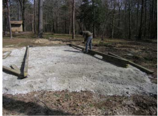
Figure D.17. Crush-and-run gravel placed on top of the ground liner to create the foundation for the stall floor. (Photo by G. W. Wood.)
