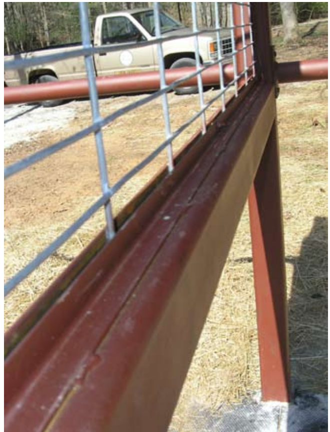
Figure D.5. Angle iron framing to secure the divider screen. (Photo by G. W. Wood.)
