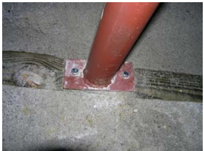
Figure D.9. Attachment of stall bars to the floor framing and center support beam timbers with \frac{3}{8} - x3-in., galvanized lag bolts (GHD if available). (Photo by G. W. Wood.)
